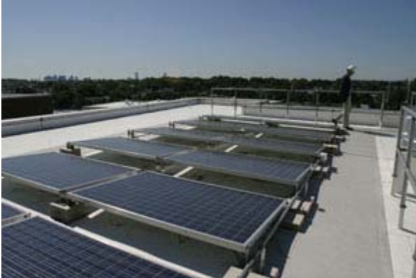
Solar arrays on Tufts' green dorm, Sophia Gordon Hall, opened in September 2006. Photo: Melody Ko/Tufts University
