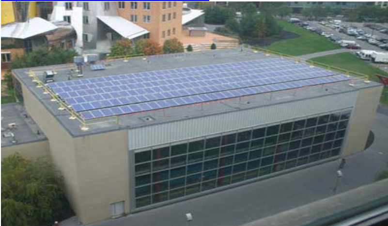
MIT's biggest array of solar panels is expected to go into service this month, producing an estimated 50,000 kWhs annually in clean energy. That's equivalent to removing 65,000 pounds of carbon dioxide from the atmosphere
